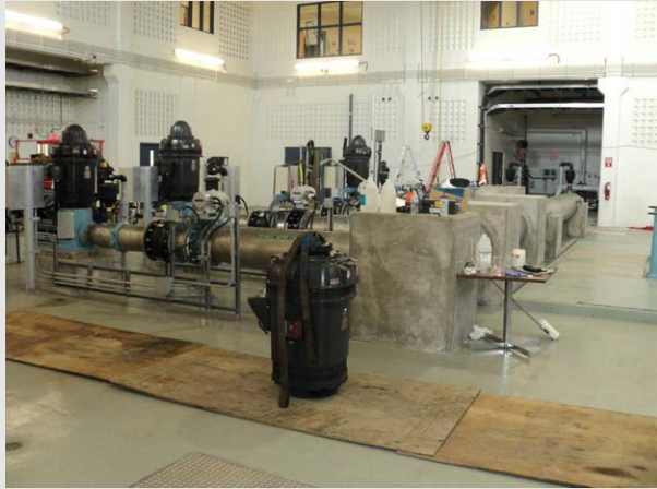
Port Hope's three remaining operating pumps
