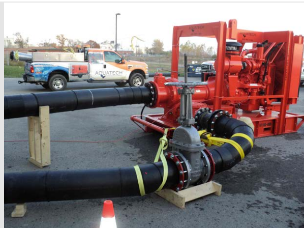
Pump showing Suction and Discharge Piping
